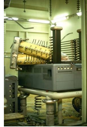
Fig. 3 1971 San Fernando Earthquake: damaged converter in Sylmar. (source: NISEE, 2009)
