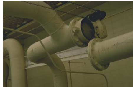
Fig. 4 1971 San Fernando Earthquake: damaged to piping at Olive View hospital power plant. (source: NISEE, 2009)
